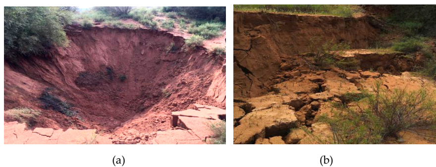
Figure 20. Field surface cracks: (a) sinking funnel; (b) step crack.
